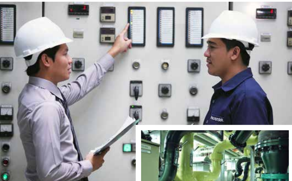
EQUIPMENT ROOM AT AYALA TOWER ONE & EXCHANGE PLAZA
